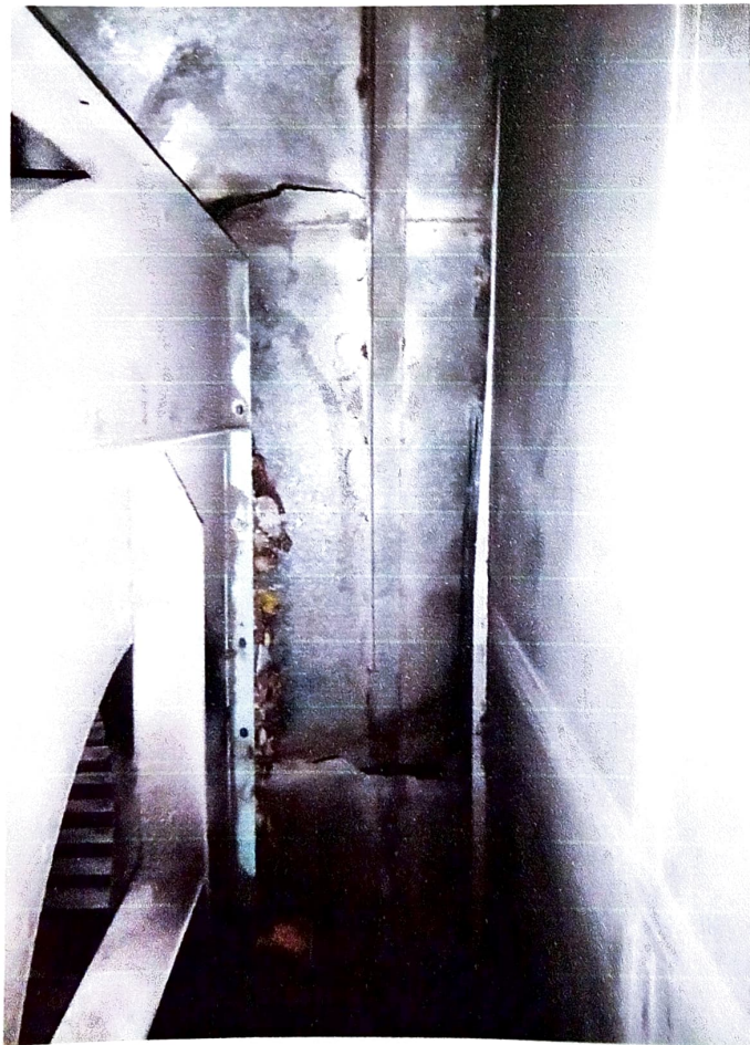
Figure 1.13: Damaged structure of AHU
