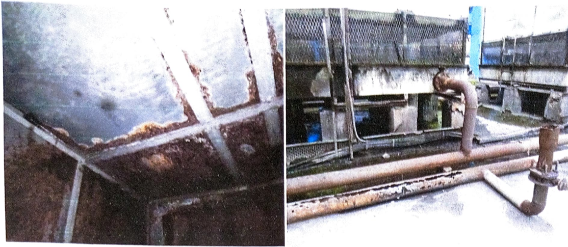
Figure 1.14: Damaged structure of AHU
