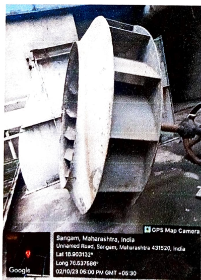
Figure 1.3: Condition of the blower wheel for air washer
