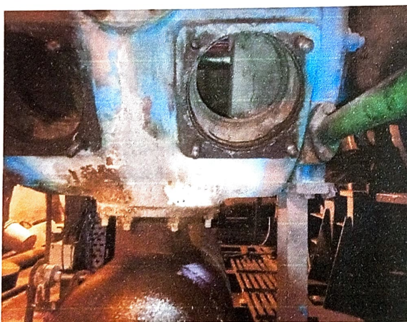
Figure 1.9: Damaged chiller assembly
